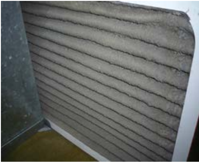
Curtis Wankel of Vesta Property Inspections in Calgary, Alberta snapped this photo of an extremely clogged filter. A filter this dirty blocks airflow and could damage your furnace.
